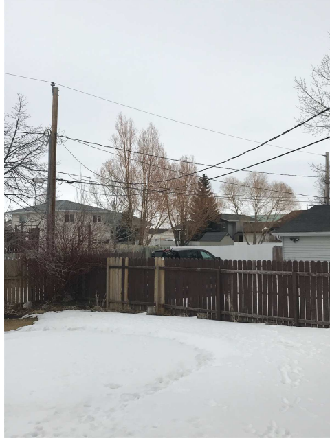
Figure 7.2 Coaxial Cables Hung From Utility Poles
