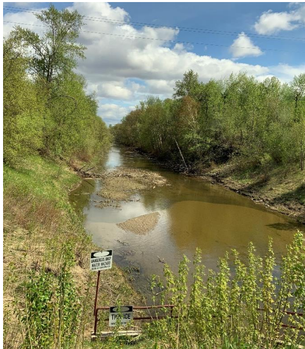
Image 3.10 The Dragline Channel showing sedimentation, May 2019
