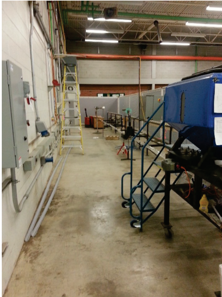
Figure A-1: Air handling system components from top-left to bottom-right: product collection box, downstream conveying line, horizontal bleed-off, upstream conveying-line, product tank and metering system.
