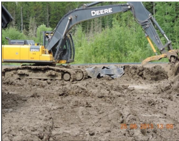
Figure C9 A large pit was dug at the spill site and then lined to provide storage for the most heavily damaged soil and plant material before it was removed (Gerbrandt 2013).
