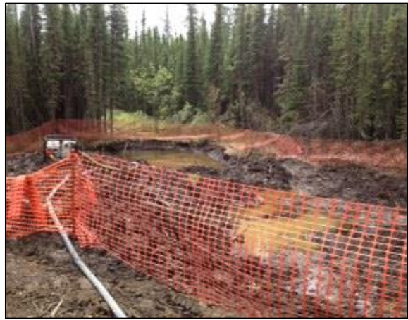
Figure C3 Alternate view of Figure 4.1 showing the area of the pipe break after heavy rain (Gerbrandt 2013).
