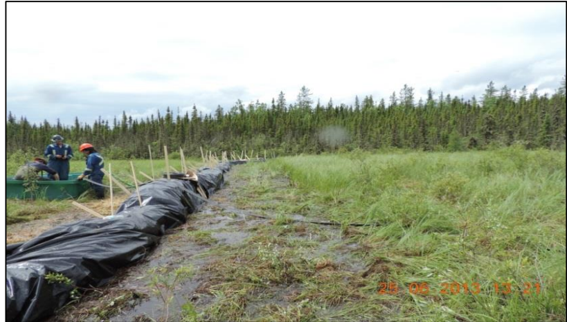
Figure C6 Hay bales at the perimeter of the spill site weighed down and covered with plastic (Gerbrandt 2013).
