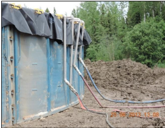
Figure C7 Produced water at the spill site was stored in this pool until it could be cleaned via reverse osmosis (Gerbrandt 2013).
