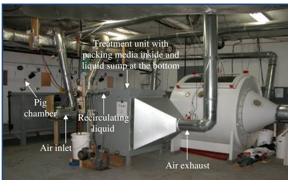
Figure 5.2 Photo of the actual set-up of the biotrickling filter unit.
