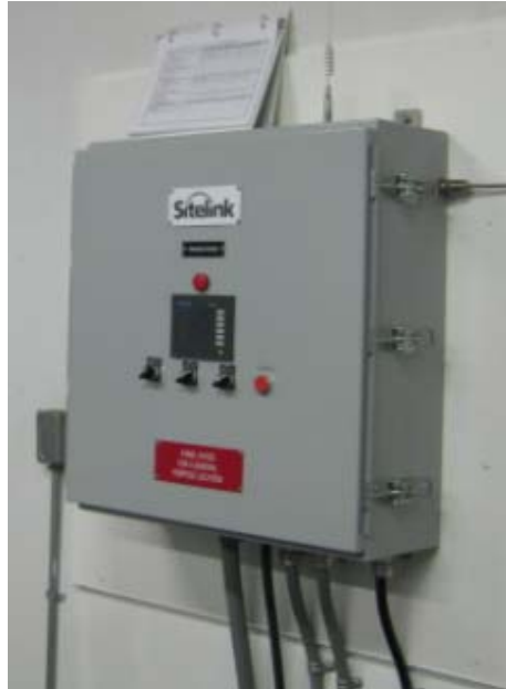
Figure 2.4 SaskWater Clarence Booster Station SCADA
