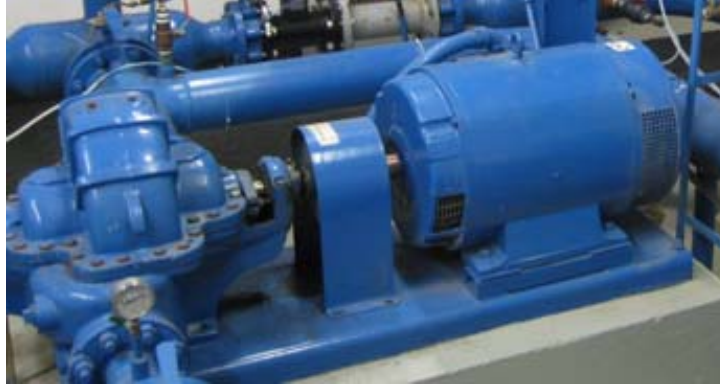
Figure 2.3 Centrifugal pump in CBS
