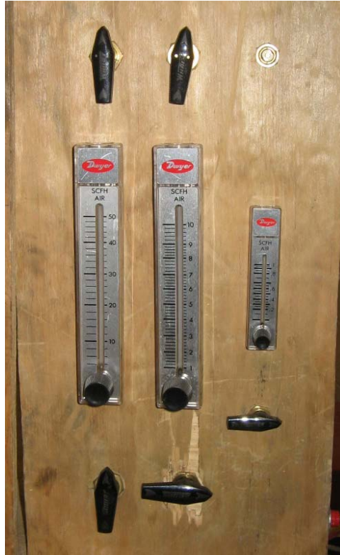
Figure 3.3. Flow meter manifold in 2006 AP design.
