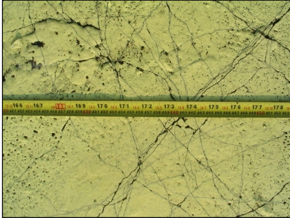
Figure 3.2. Surface fractures in the Phase I block.
