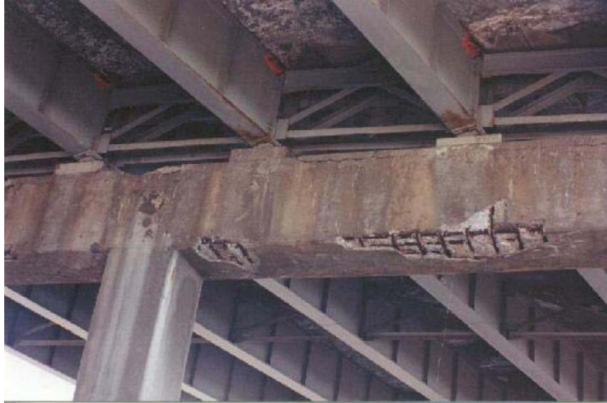
Figure 1.1 Corrosion of a cross girder that supports the main bridge deck (Thompson and Yunovich, 2003)
