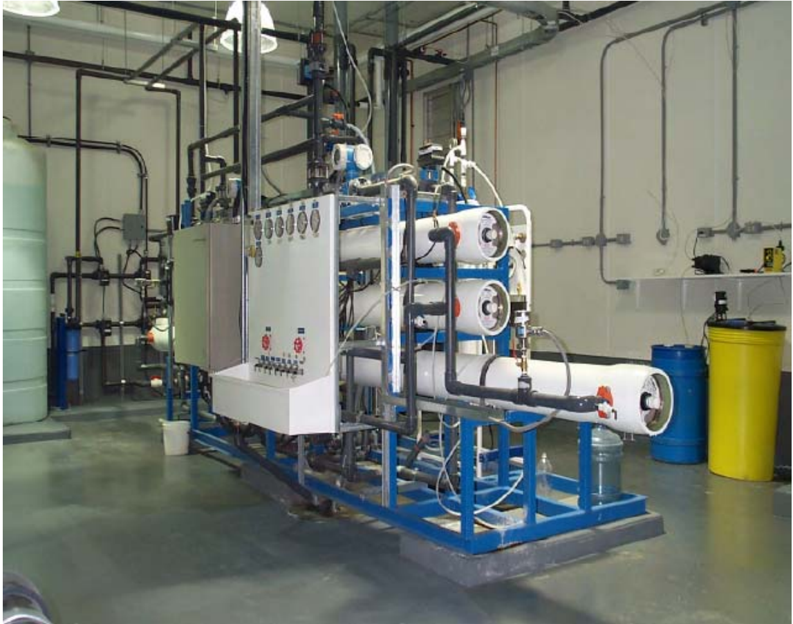
Figure 5.13 Reverse Osmosis system in the Yellow Quill Water Treatment Plant.
