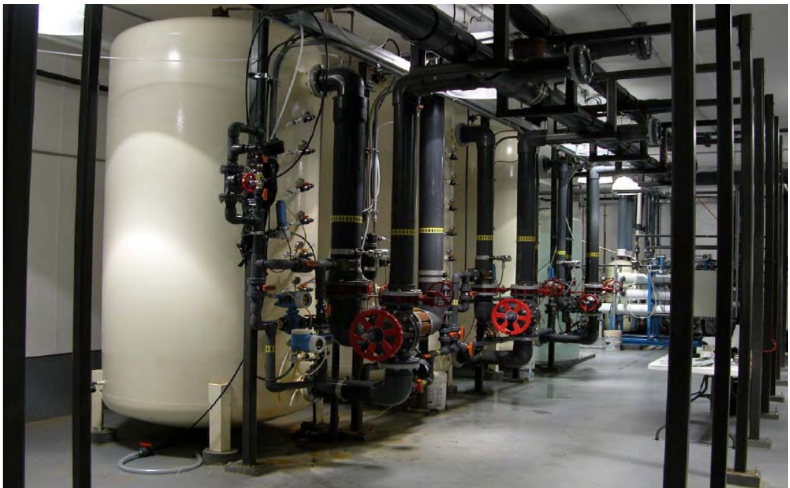
Figure 5.12 Biological filter system in the Yellow Quill Water Treatment Plant.
