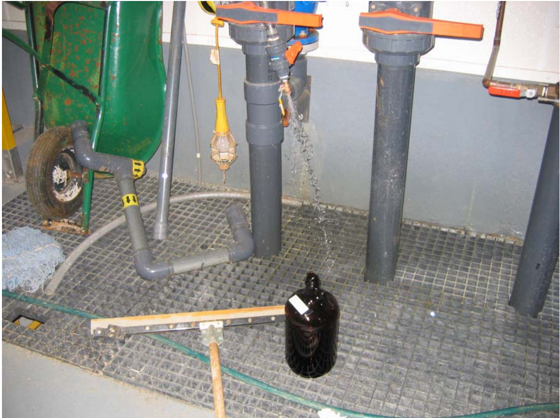
Figure 5.14 Sampling bottle used at the Yellow Quill Water Treatment Plant.
