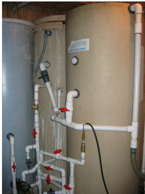
Figure 5.30 Slow sand filtration and biological activated carbon treatment vessels.
