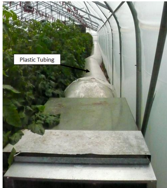
Figure 4.7 Plastic heating duct in the greenhouse (water-air heat exchanger in the front)
