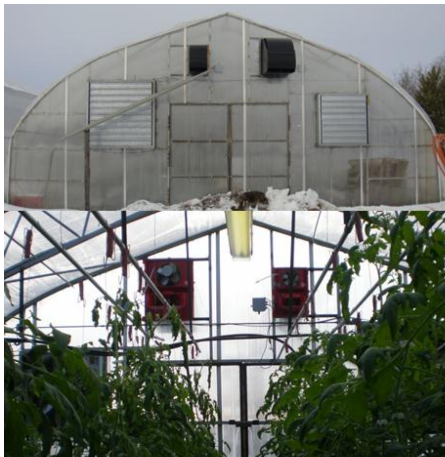
Figure 4.9 Picture of heat exchangers setup
