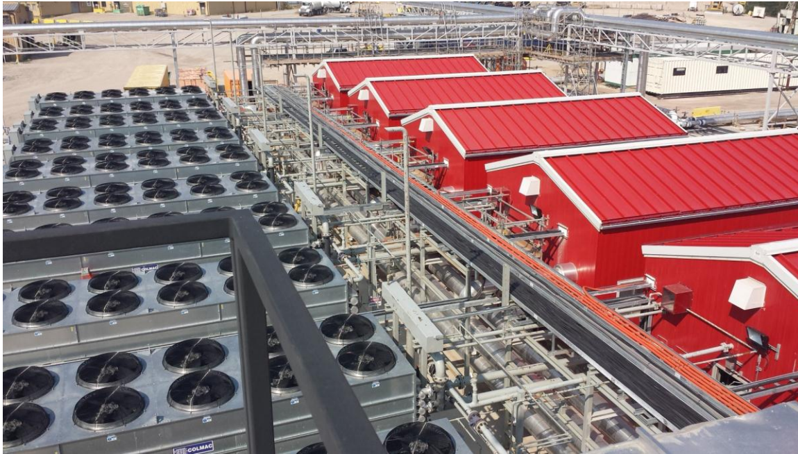
Figure 3-2 Cigar Lake Modular Refrigeration Plant with Five Modules and Condensers
