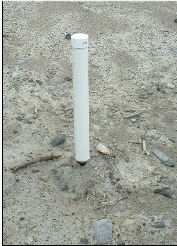
(b) Protective covering over gas ports
