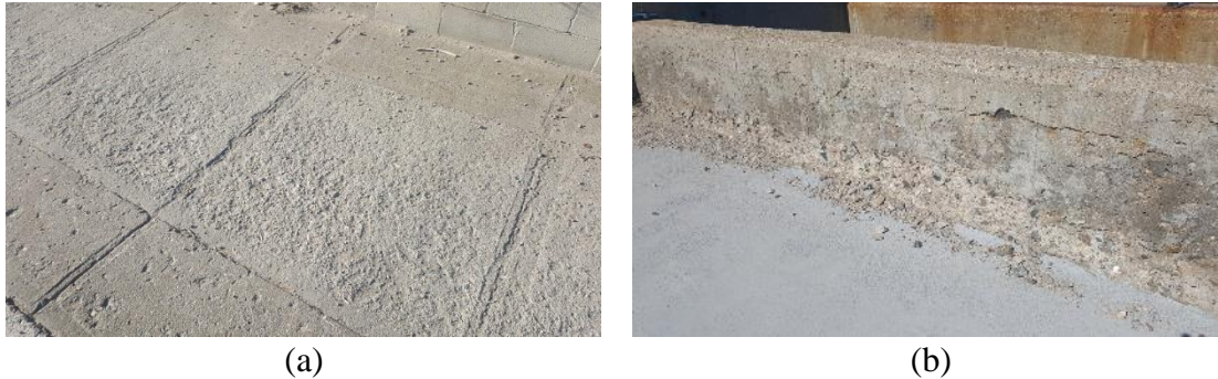
Figure 2.2 Effect of freezing and thawing in concrete: (a) Scaling, and (b) Spalling
