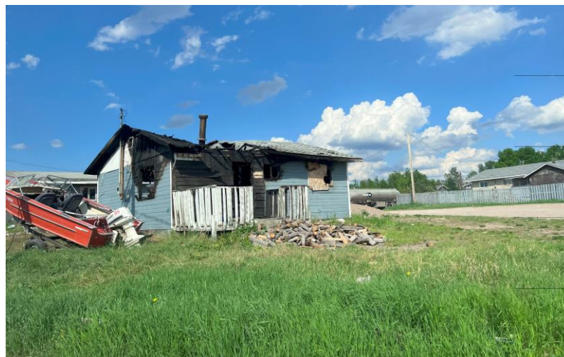
Figure 3.5 Residential fire incident caused by a woodstove, captured during a community visit in June 2023 (author’s own captured).
