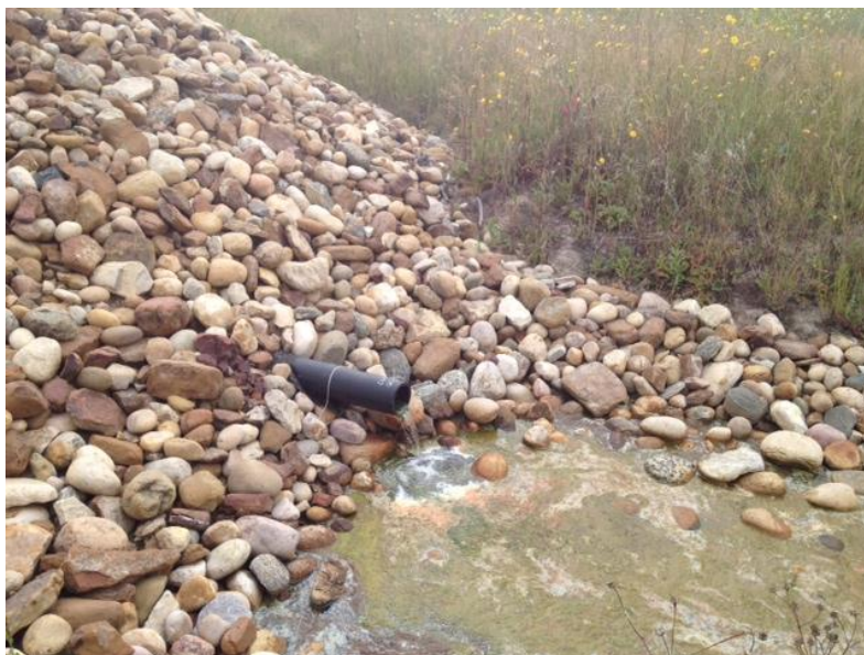
Figure 3.7: Underdrain discharge at SWSS Cell 46
