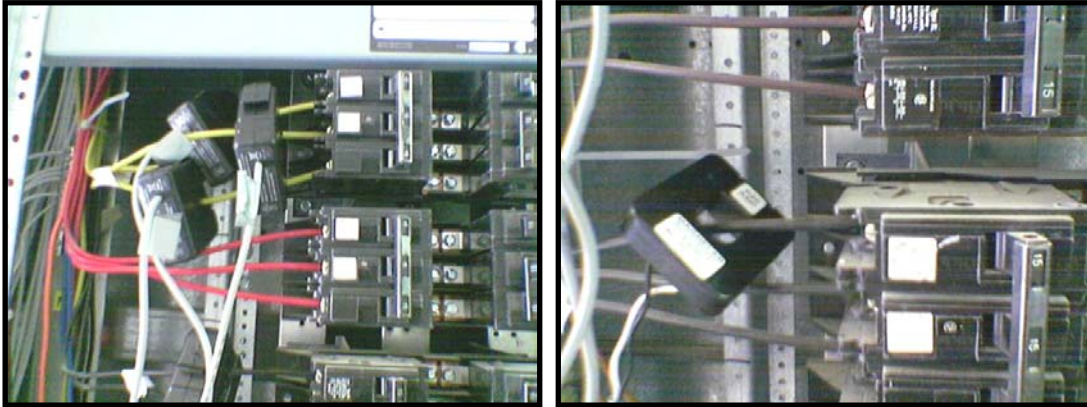
Figure 4.1 Current sensors hooked up to the wire in the electrical panel
